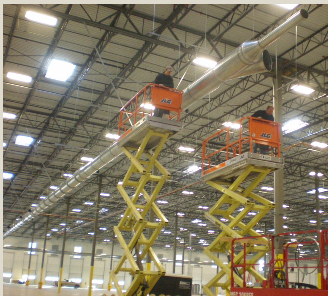
Two Wilson Sheet Metal employees on lifts install 24-inch Quick-Fit duct at an Atlanta furniture manufacturing facility.
